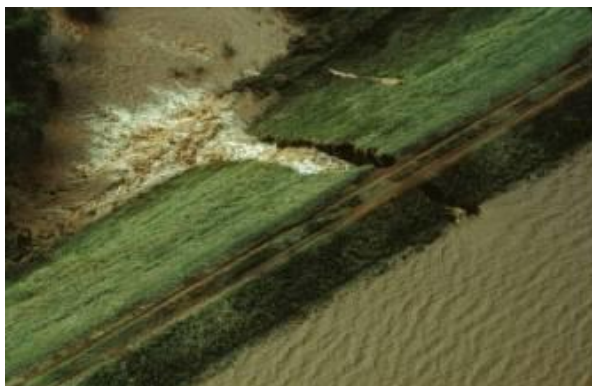
Figure 1. Internal erosion of USDA-NRCS structure
